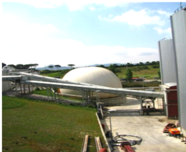
Figure 3. Anaerobic Digestion Facility, Spain
